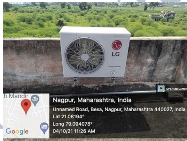
AC Condenser exposed to direct sunlight
