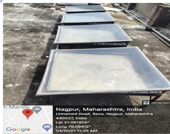
Solar Pv System for Water Distillation System
